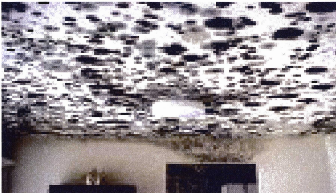
MOLD GROWTH ON A CEILING
