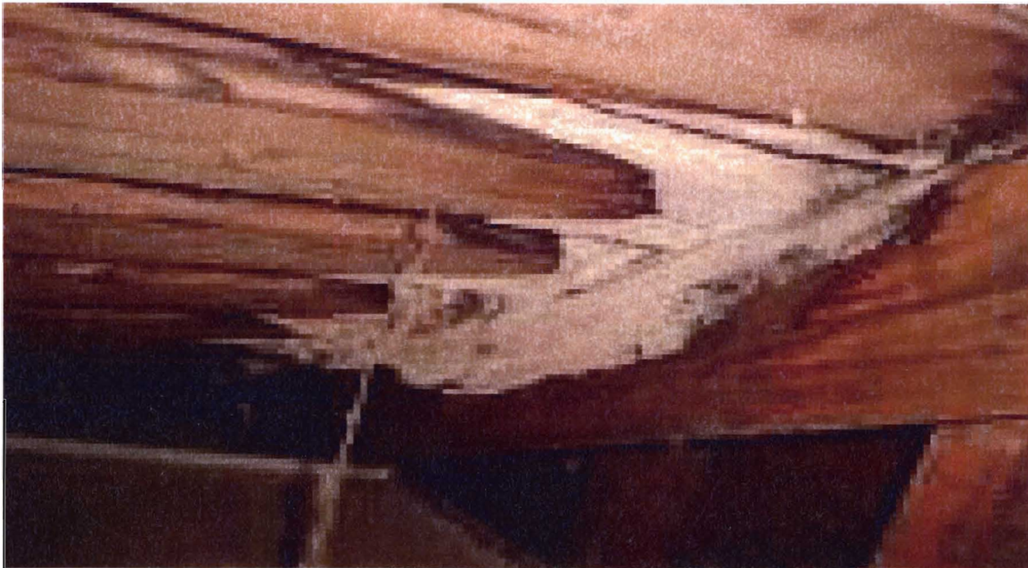
MOLD GROWTH INSIDE AN ATTIC
