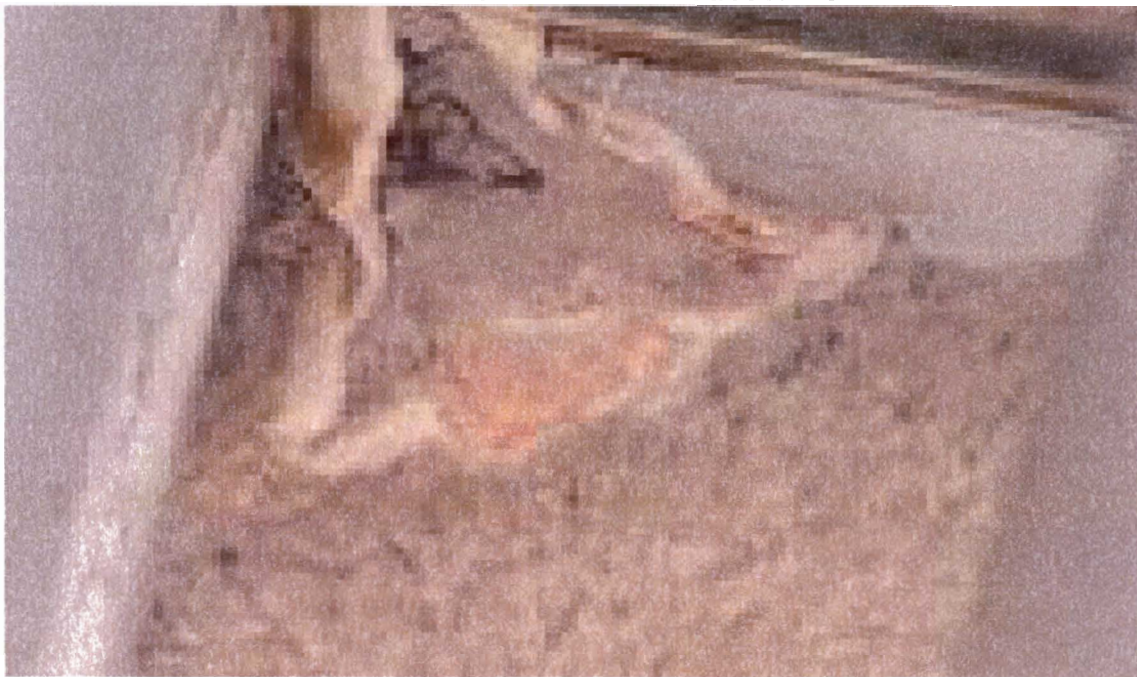
MOLD MUSHROOMS GROWING IN A WALL
