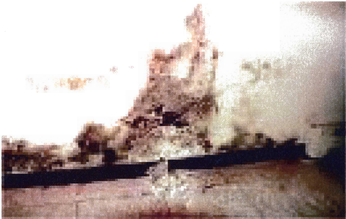
MOLD ON A WALL AND FLOOR IN A ROOM
